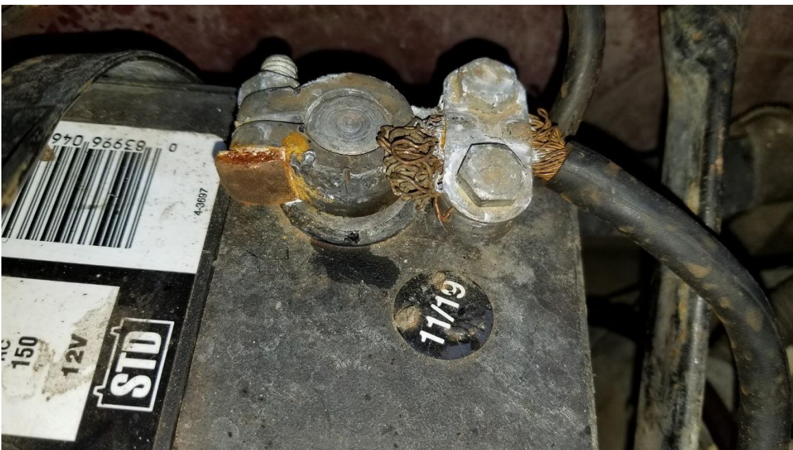
Poor battery terminals
