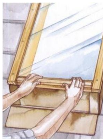
Lay the glass into the skylight frame and secure it with redwood stops. Use a beveled stop for the bottom piece.
