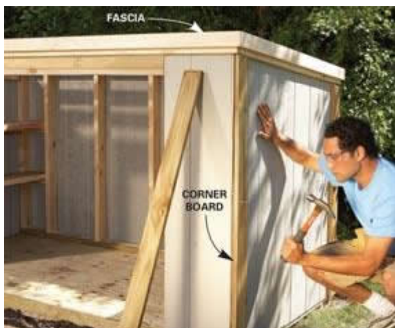
PHOTO 7: NAIL ON THE TRIM
