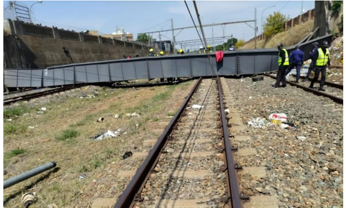
Pedestrian bridge collapse in Johannesburg, 2023
