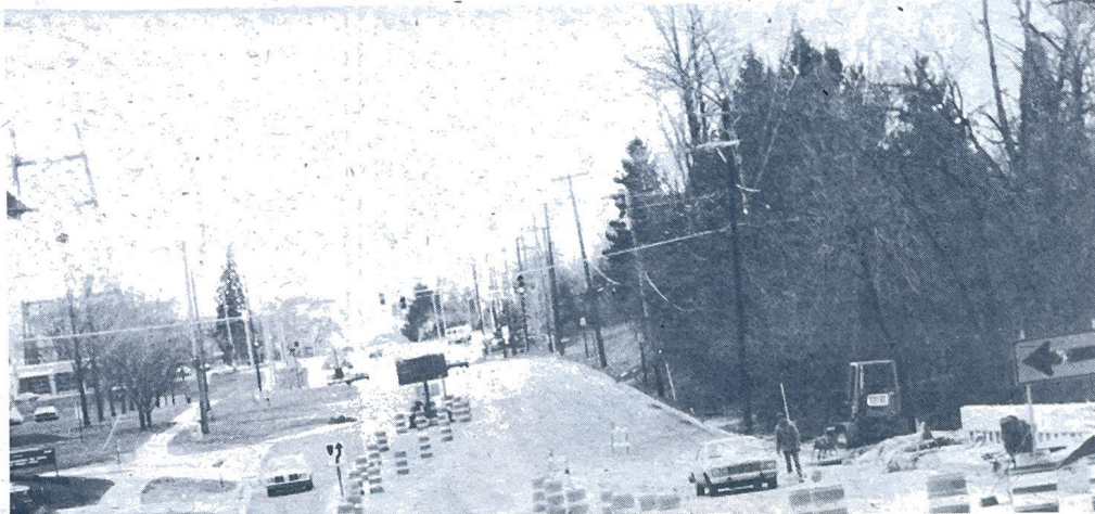
Workmen conclude construction on the new Lahser Road bridge south of SHS. (Photo by Brian Dubanik)
